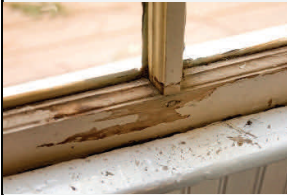
Flaking paint on a window sill—assume it contains lead paint unless testing indicates otherwise
