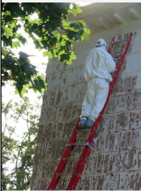
Wet scraping/stabilization (removal of loose and flaking paint) performed by a licensed deleading contractor
