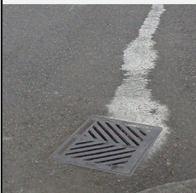
Storm Drains- Frequently check hydraulic lines for trash compactors that are near storm drains
